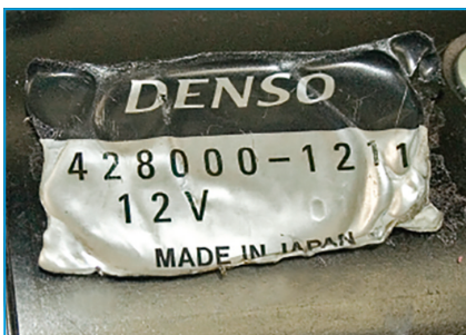
ID tag has been overheated and has shrunk. This is a sign of excessive heat.
