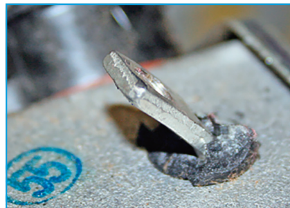
Damage to the terminal could cause ground contact with housing.
